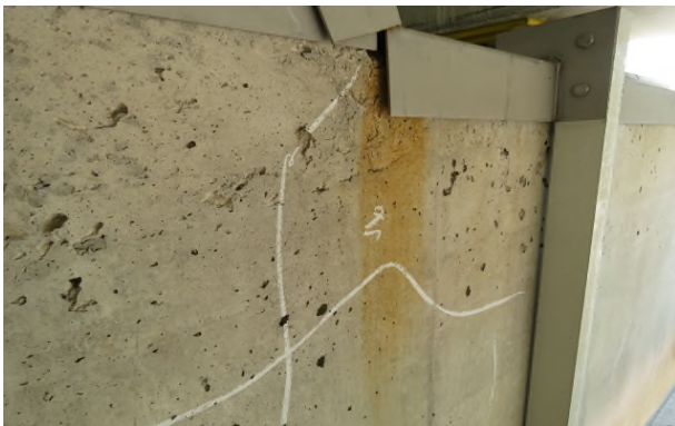
⑰ 균열 (0.3mm미만) cw=0.1mm / 0.4m
