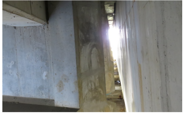
⑤ 균열 (0.3mm미만) cw=0.2mm / 0.5m (4EA) (보수완료)
