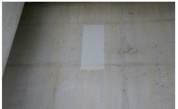
㉔ 균열 (0.3mm미만) cw=0.05mm / 0.5m (보수완료)
