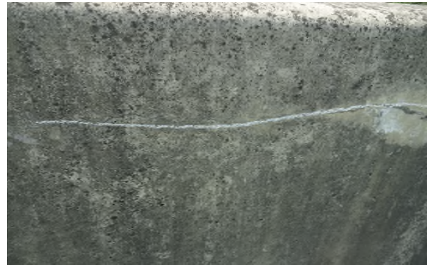
⑭ 균열 (0.3mm미만) cw=0.1mm / 0.7m
