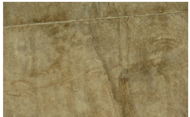
⑳ 균열 (0.3mm미만) cw=0.2mm / 2.5m
