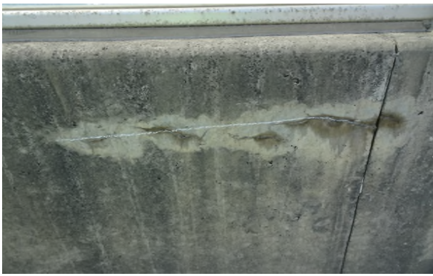
㉔ 균열 (0.3mm미만) cw=0.2mm / 0.6m
