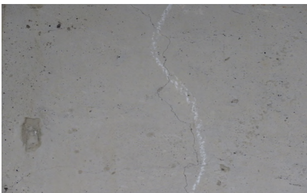
⑨ 균열 (0.3mm미만) cw=0.2mm / 1.0m
