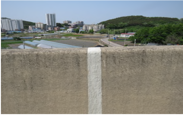
① 균열 (0.3mm미만) cw=0.1mm / 1.5m (보수완료)
