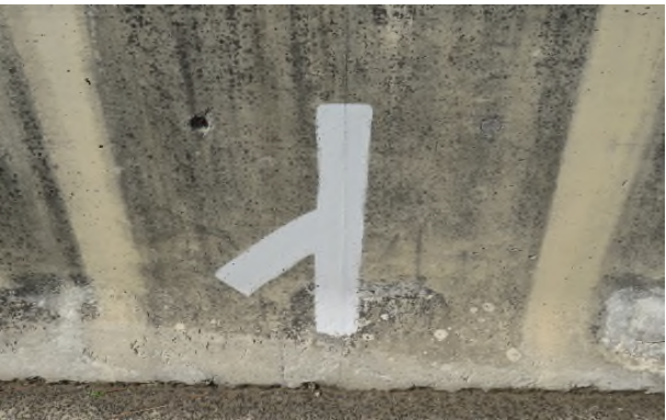
⑬ 균열 (0.3mm미만) cw=0.1mm / 0.5m (보수완료)
