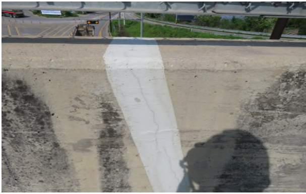
⑨ 균열 (0.3mm미만) cw=0.1mm / 0.5m (보수완료)
