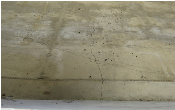
⑰ 균열 0.2mm / 0.4m
