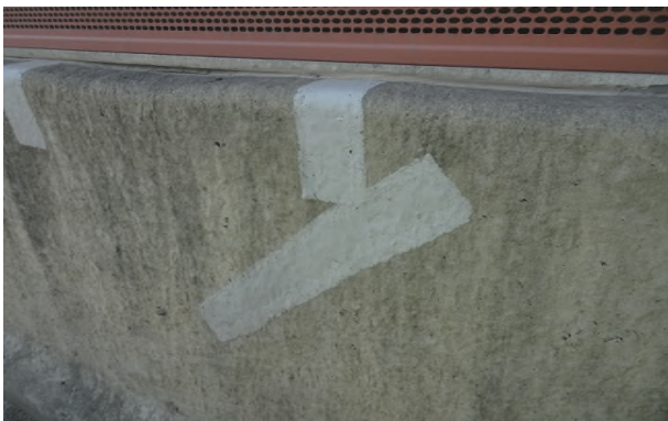
⑯ 균열 (0.3mm미만) cw=0.1mm / 0.2m (5EA) (보수완료)
