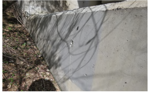
③ 균열 (0.3mm미만) cw=0.2mm / 0.9m (보수완료)
