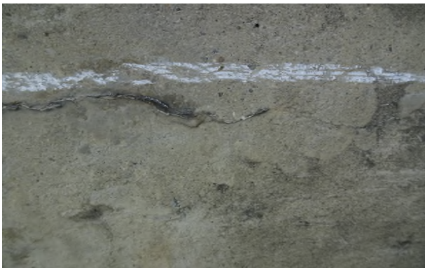
㉑ 균열 (0.3mm미만) cw=0.2mm / 1.0m
