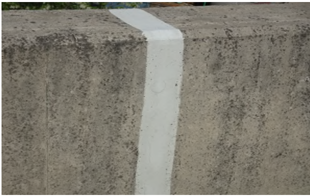
③ 균열 (0.3mm미만) cw=0.1mm / 0.5m (2EA) (보수완료)
