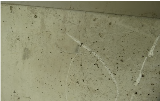
⑭ 균열 (0.3mm미만) cw=0.1mm / 0.6m
