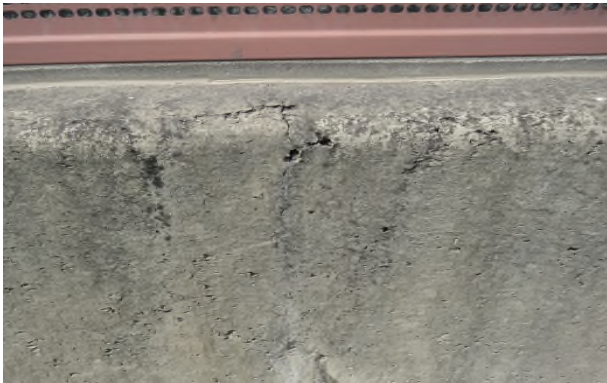
㉔ 균열 (0.3mm미만) cw=0.1mm / 0.4m (4EA)
