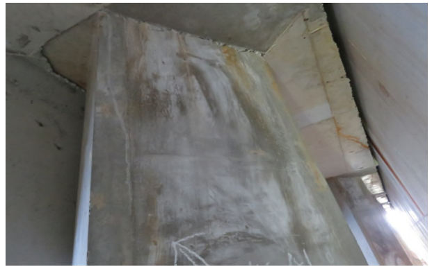
⑦ 균열 (0.3mm미만) cw=0.2mm / 0.5m (5EA) (보수완료)
