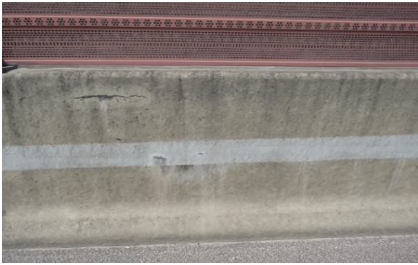
① 균열 (0.3mm미만) cw=0.2mm / 2.0m (4EA) (보수완료)
