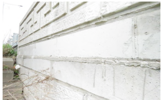
⑮ 균열 (0.3mm미만) cw=0.1mm / 1.0m (3EA) (보수완료)
