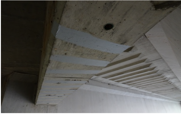
③ 균열 0.2mm / 0.6m (13EA) (보수완료)
