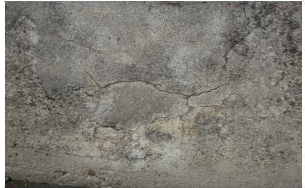
④ 망상균열 (0.3mm미만) cw=0.1mm / 0.6m x 0.5m
