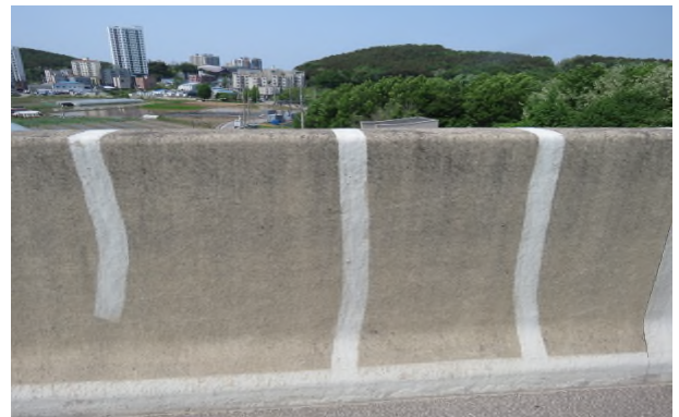
④ 균열 (0.3mm미만) cw=0.2mm / 1.5m (12EA) (보수완료)
