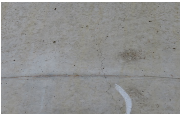
⑯ 균열 (0.3mm미만) cw=0.1mm / 2.5m
