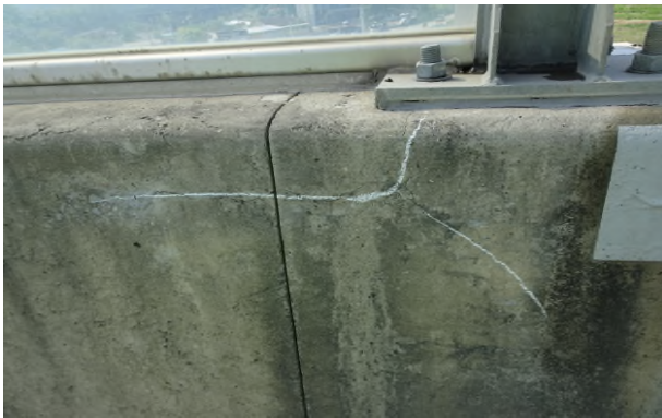
②② 균열 (0.3mm미만) cw=0.2mm / 0.5m
