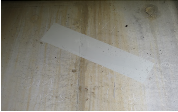
⑨ 균열 (0.3mm미만) cw=0.1mm / 0.5m (보수완료)
