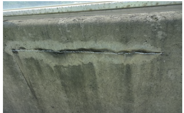
②③ 균열 (0.3mm미만) cw=0.2mm / 0.8m
