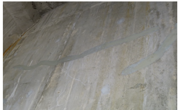
⑦ 균열 0.5mm / 1.5m (보수완료)
