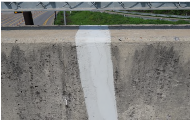
⑪ 균열 (0.3mm미만) cw=0.1mm / 0.3m (4EA) (보수완료)
