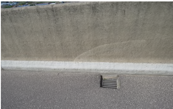
③ 균열 (0.3mm미만) cw=0.2mm / 5.0m (보수완료)
