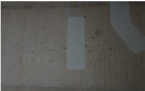
⑲ 균열 (0.3mm미만) cw=0.02mm / 0.2m (보수완료)
