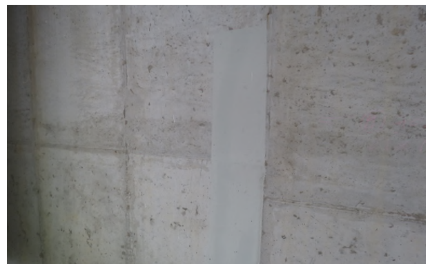
⑧ 균열 (0.3mm미만) cw=0.1mm / 1.5m (보수완료)
