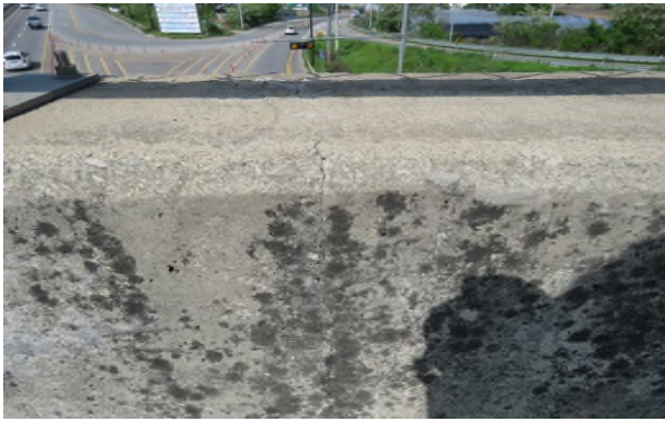
㉟ 균열 (0.3mm미만) cw=0.1mm / 1.5m
