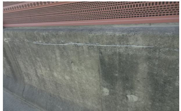
㉓ 균열 (0.3mm미만) cw=0.2mm / 1.0m
