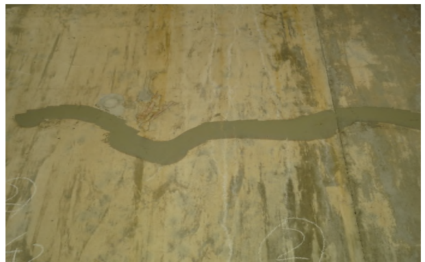
② 균열 0.5mm / 1.4m (보수완료)
