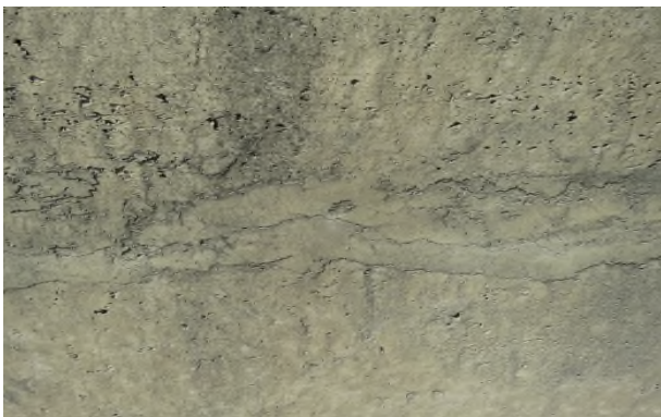
⑦ 균열 (0.3mm미만) cw=0.1\text{mm} / 4.0m
