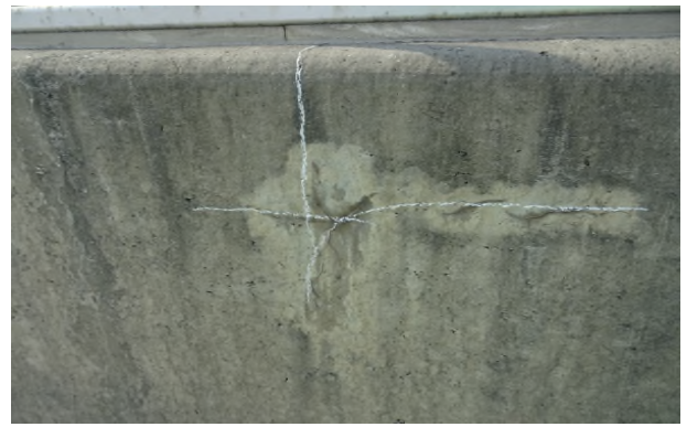
㉕ 균열 (0.3mm미만) cw=0.1mm / 0.6m
