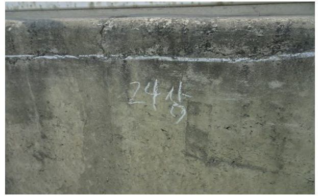
⑱ 균열 (0.3mm미만) cw=0.2mm / 2.0m
