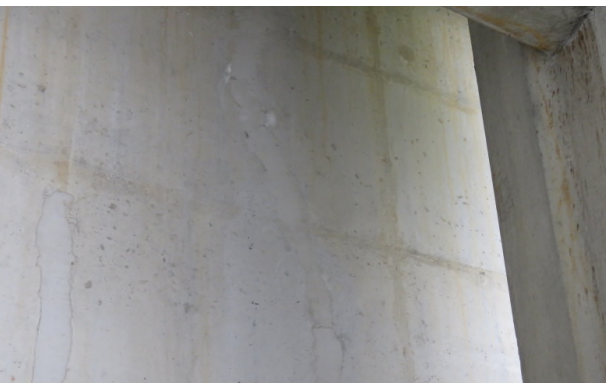
㉓ 균열 (0.3mm미만) cw=0.2mm / 2.5m (보수완료)
