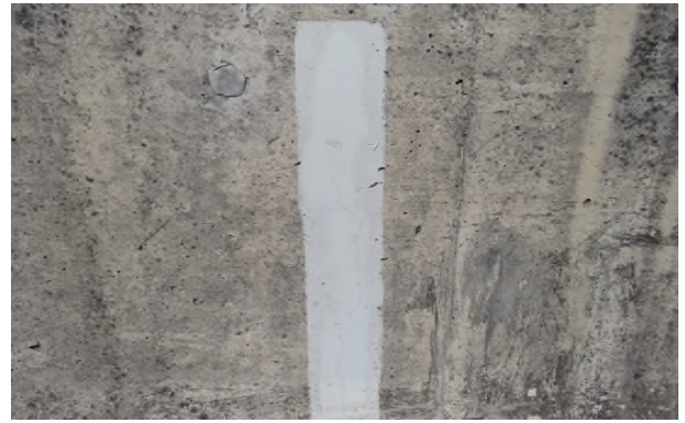
⑩ 균열 (0.3mm미만) cw=0.1mm / 0.5m (보수완료)
