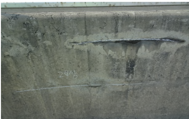
②④ 균열 (0.3mm미만) cw=0.2mm / 0.8m (3EA)
