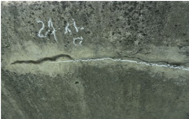
⑬ 균열 (0.3mm미만) cw=0.2mm / 1.3m
