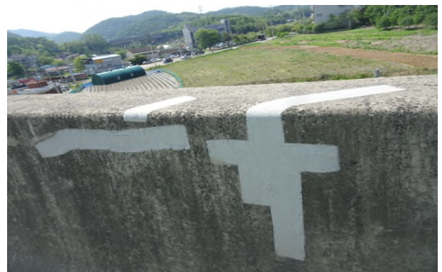
⑧ 균열 (0.3mm미만) cw=0.2mm / 0.3m (보수완료)
