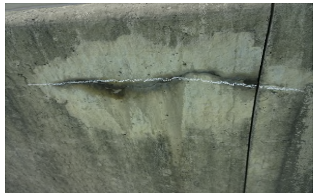
②⑤ 균열 (0.3mm미만) cw=0.2mm / 0.6m
