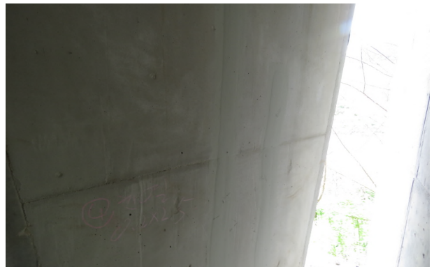
④ 균열 (0.3mm미만) cw=0.2mm / 2.5m (보수완료)
