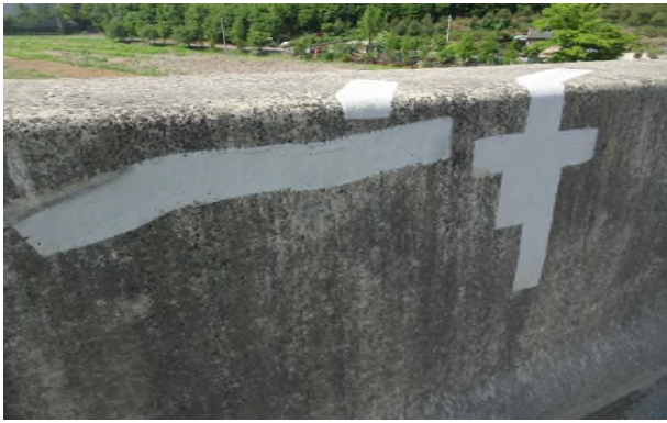
⑨ 균열 (0.3mm미만) cw=0.1mm / 0.4m (보수완료)
