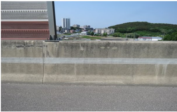
③ 균열 (0.3mm미만) cw=0.2mm / 22.0m (보수완료)
