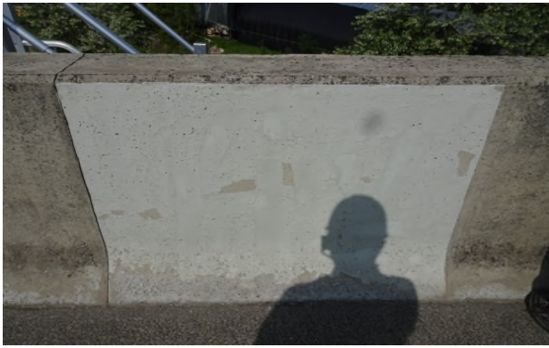
① 망상균열 (0.3mm미만) cw=0.2mm / 1.2m x 0.4m (보수완료)
