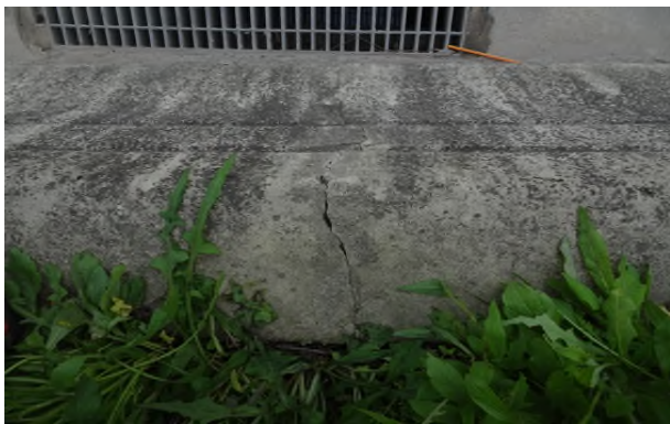
⑩ 균열 cw=0.2mm / 0.9m
