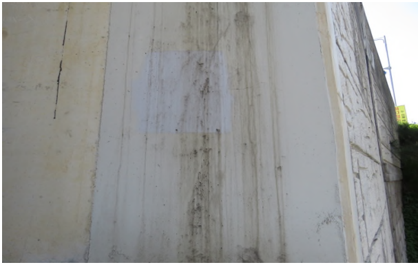
⑲ 망상균열 (0.3mm미만) cw=0.1mm / 1.0m x 2.5m (보수완료)
