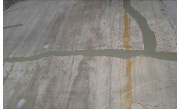
⑭ 균열 0.5mm / 1.4m (보수완료)
