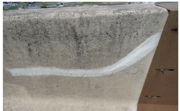
⑥ 균열 (0.3mm미만) cw=0.2mm / 1.0m (보수완료)
