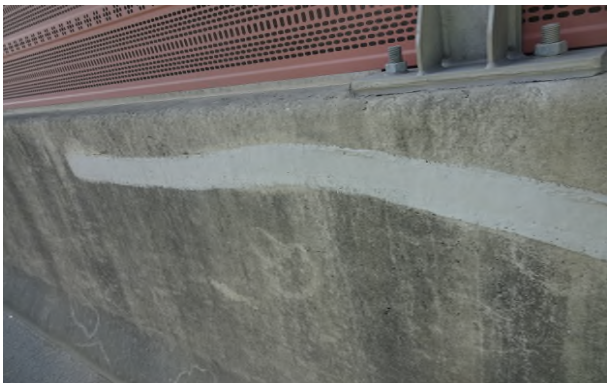
㉒ 균열 (0.3mm미만) cw=0.1mm / 0.4m (보수완료)
