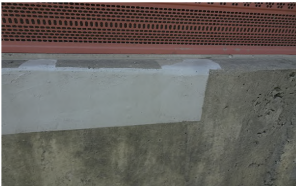
⑬ 균열 (0.3mm미만) cw=0.1mm / 4.0m (보수완료)
