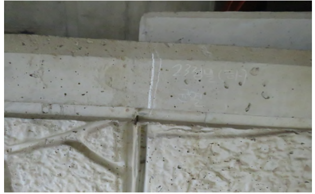
⑳ 균열 (0.3mm미만) cw=0.1mm / 0.5m
