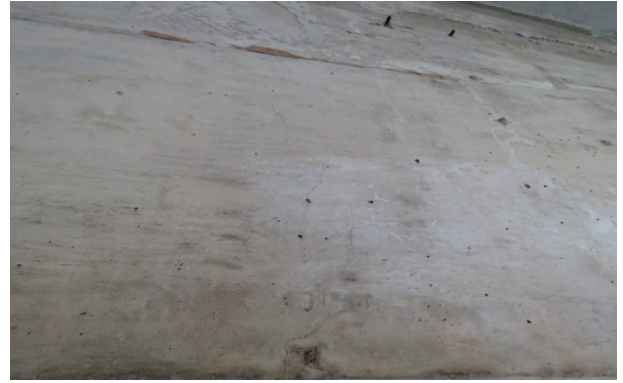
㉒ 균열 0.2mm / 0.4m (3EA)
