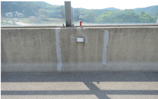
⑰ 균열 0.2mm / 1.5m (보수완료)
