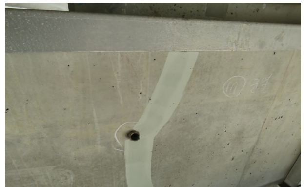
⑰ 균열 (0.3mm미만) cw=0.05mm / 0.5m (보수완료)
