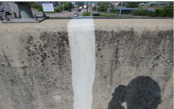
⑦ 균열 (0.3mm미만) cw=0.2mm / 1.5m (보수완료)
