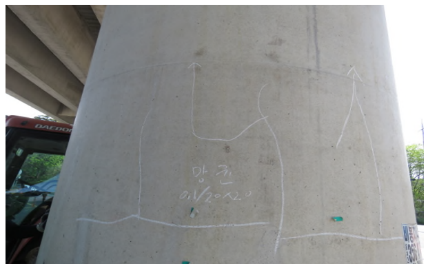
⑰ 망상균열 (0.3mm미만) cw=0.1mm / 2.0m x 2.0m
