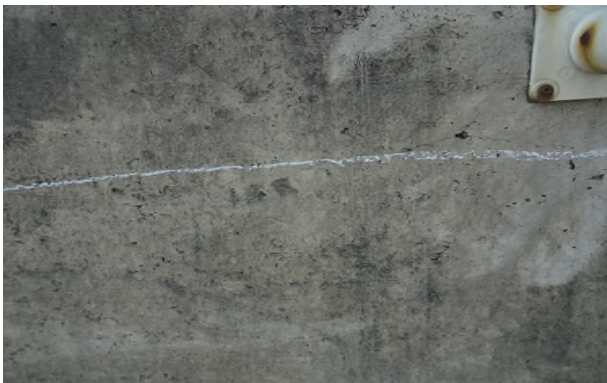
⑲ 균열 (0.3mm미만) cw=0.2mm / 1.0m
