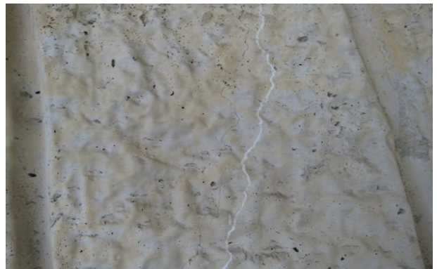
⑪ 균열 (0.3mm미만) cw=0.1mm / 0.6m
