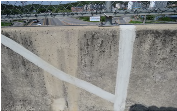
③ 균열 (0.3mm미만) cw=0.1mm / 2.0 m(보수완료)
