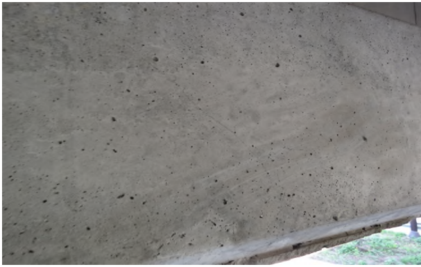
① 균열 (0.3mm미만) cw=0.1mm / 0.1m (3EA)
