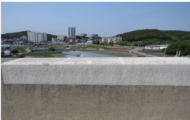
⑤ 균열 (0.3mm미만) cw=0.1mm / 0.5m (5EA) (보수완료)
