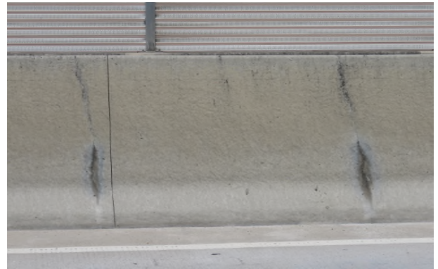
⑧ 균열 0.2mm / 1.4m (5EA) (보수완료)
