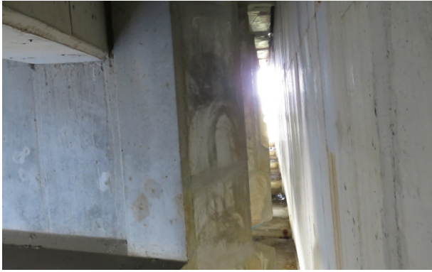
④ 균열 (0.3mm미만) cw=0.2mm / 0.5m (5EA) (보수완료)
