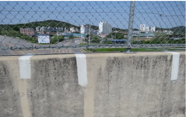
⑤ 균열 (0.3mm미만) cw=0.1mm / 0.3m (4EA) (보수완료)
